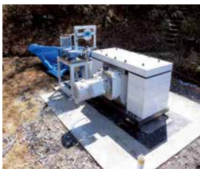
Figure 7.2. Continuous CO 2 monitoring system deployed in Canada, PI Tsuji with JOGMEC.
